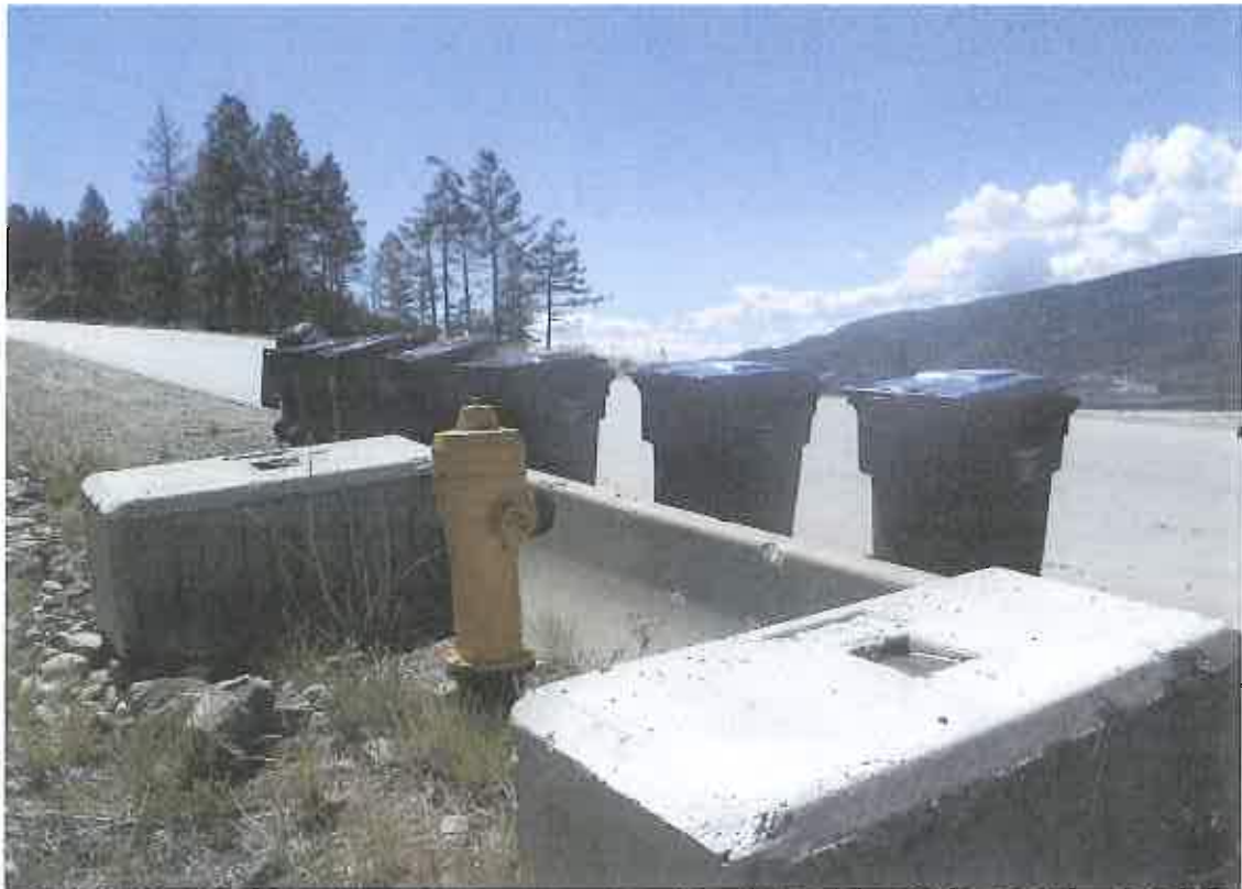
Fire Hydrant Lochview Road
